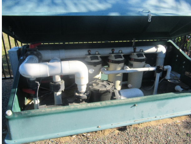
Mechanical equipment - overview
