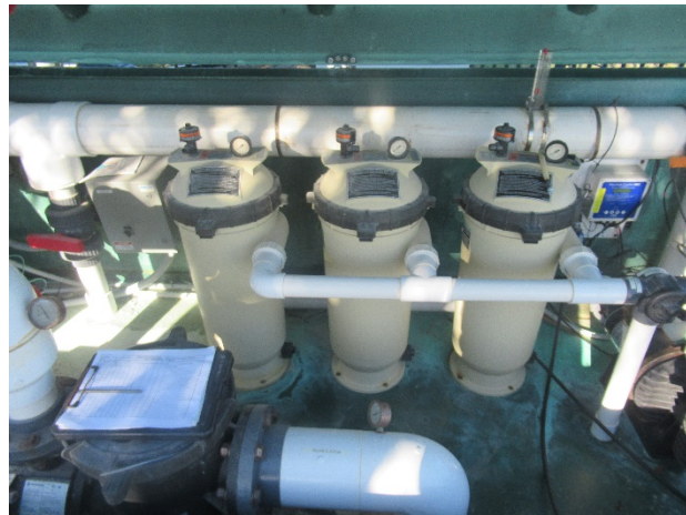
Mechanical equipment - overview
