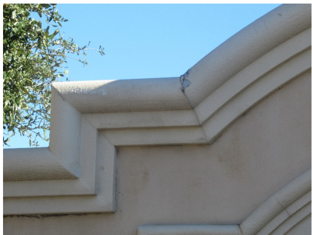
Monument signage – minor deterioration of the stucco coatings evident
