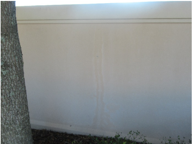
Perimeter walls – deterioration of the paint finishes as well as cracks evident
