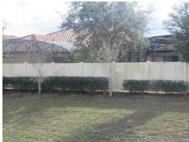
Vinyl fences – deterioration of the vinyl fences evident
