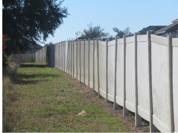
Vinyl fences – leaning sections and deterioration of the vinyl evident
