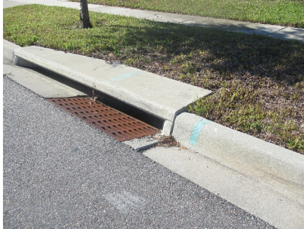
Catch basins – minor settlement evident
