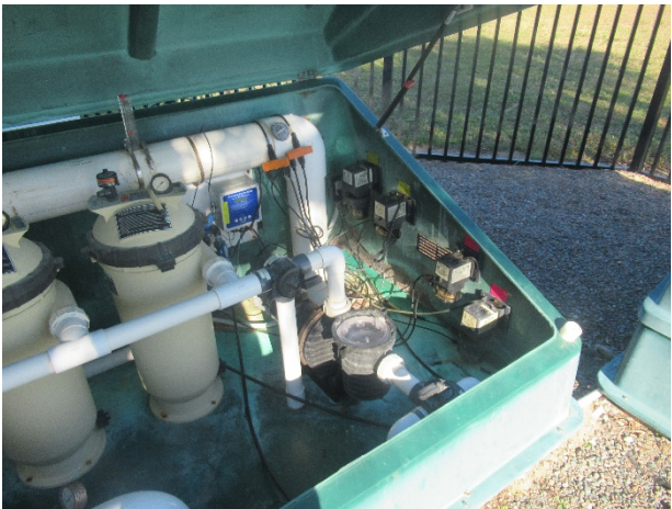
Mechanical equipment - overview
