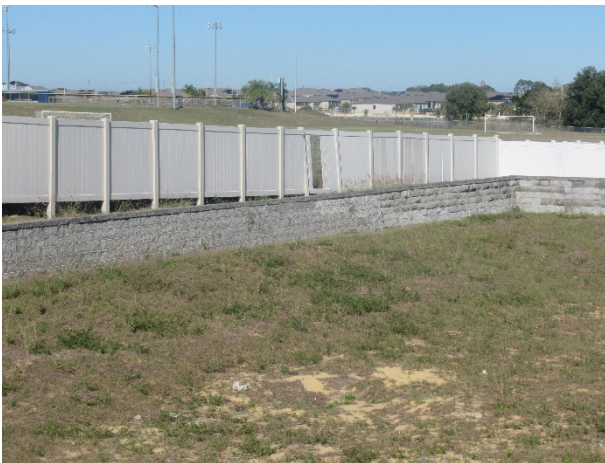
Vinyl fences – damage evident
