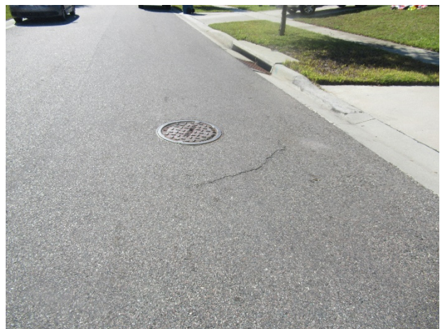
Asphalt pavement streets – isolated cracks evident
