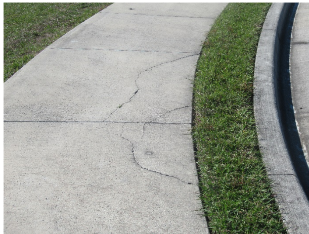
Concrete sidewalks – cracks evident
