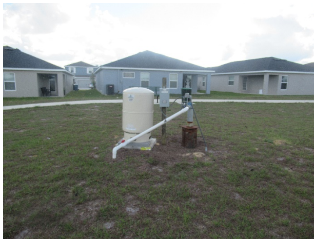
Irrigation pumps - overview
