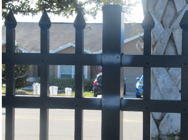
Aluminum fences – deterioration of the paint finishes evident
